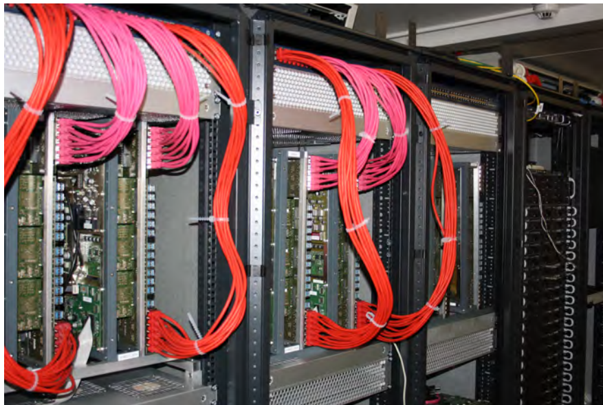
Figure 5: The Wafer Modules that are currently installed into the NM-PM1 installation racks
